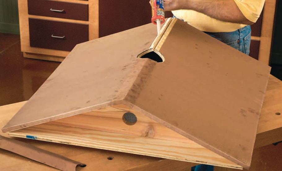
Use an outdoor-rated construction adhesive to attach the formed copper panels to the roof. Glue the large panels down first, then the ridges.
